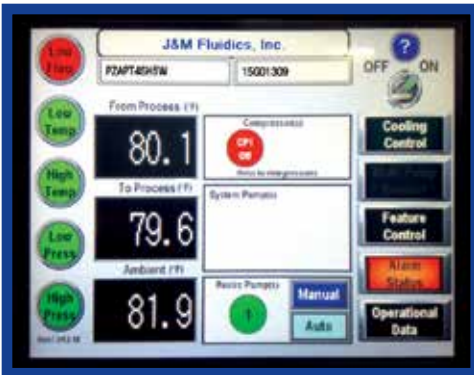
● Chiller Main Operating Screen
