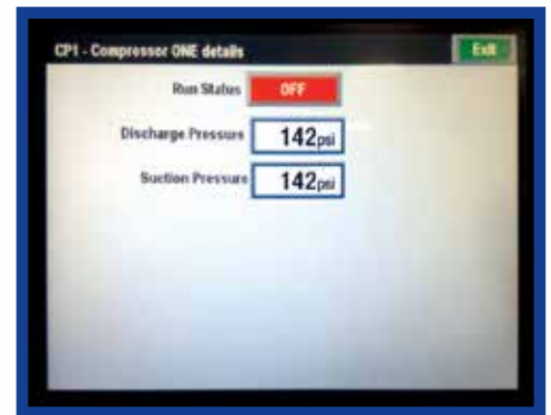
● Compressor Operation Status and Pressures
